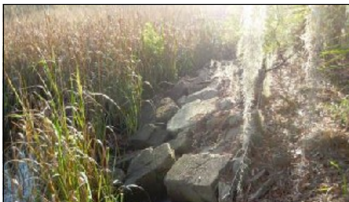
A concrete rip-rap placed along the bottom of a slope helps to stabilize the bank as adjacent uplands removal action is completed. (SOURCE: (1/23/2013 PRP response letter).
