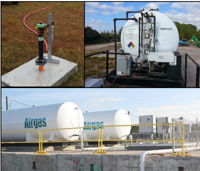
Top left: Typical sparge well. Top right: Portable CO 2 sparging system. Bottom: 50-ton CO 2 storage tanks. Images are from Figure 2-6 of the CO 2 Sparging Phase 1 Report (June 20, 2014), prepared by Mutch Associates, LLC.
